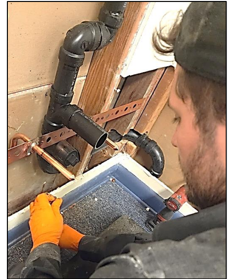
Getting a new classroom and art room ready for students started with cutting into walls to add hand-washing sinks.
